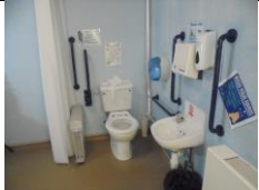
Soap dispenser and hand drying facility too high
