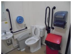
Grab rail missing from one side of sink/ mirror and coat hooks too high
